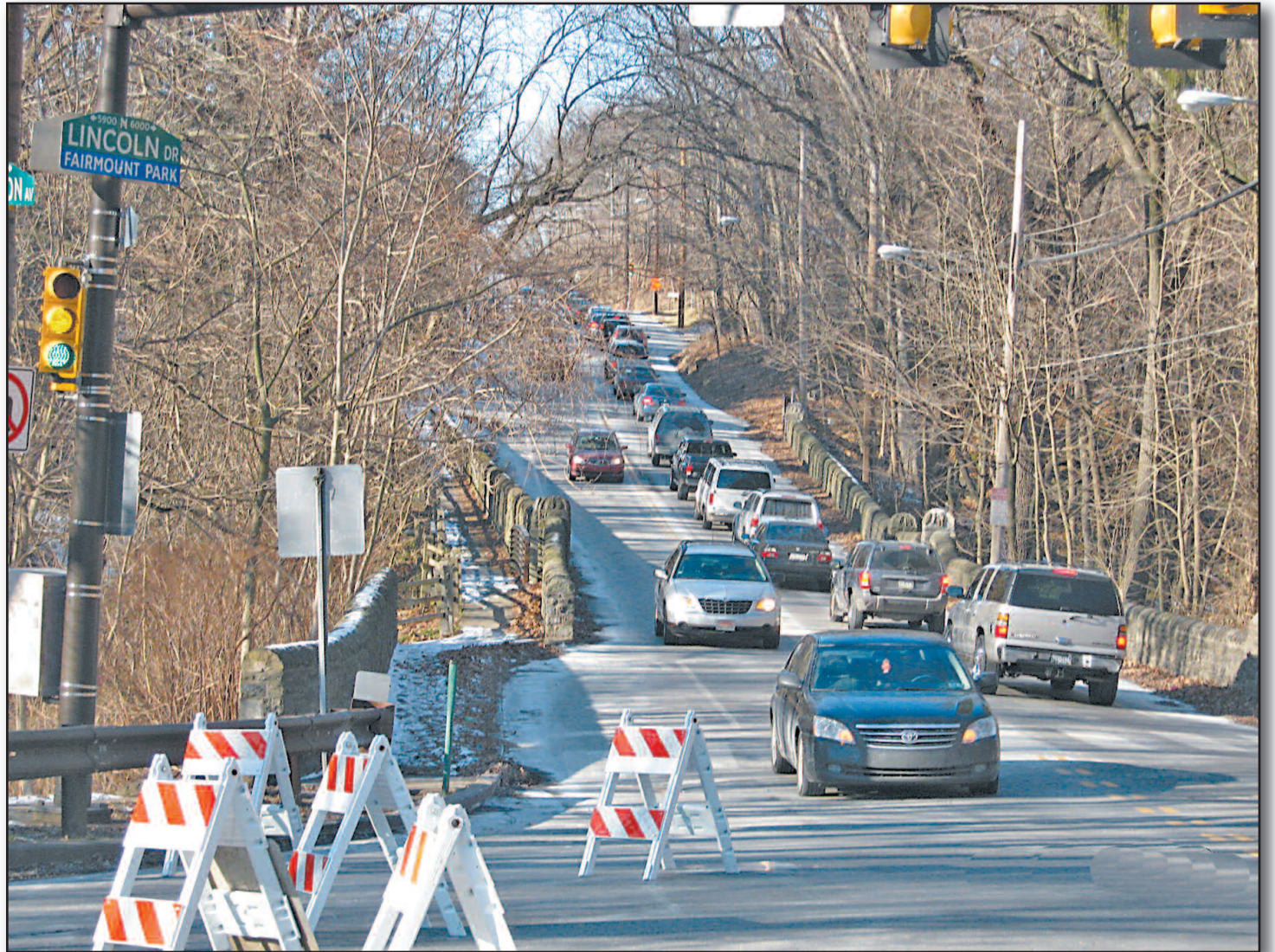
Cars streamed off Lincoln Drive onto Wissahickon Avenue all day Saturday as motorists heading downtown were forced to take other routes due to the Streets Department's upkeep and repair work on the Drive between Rittenhouse Street and Ridge Avenue. The announcement of the work and the ensuing detours was not made until last Thursday.
